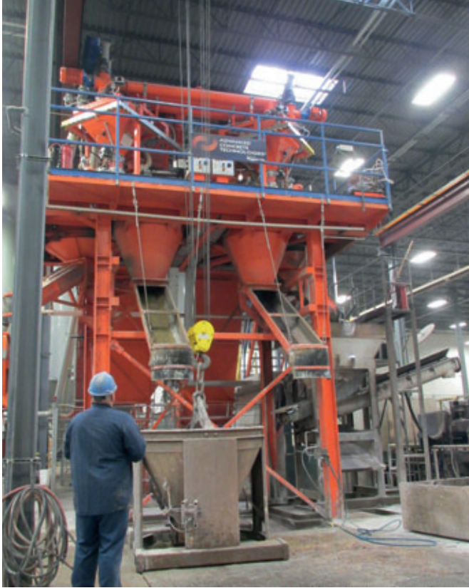
Figure 8 -- An operator remotely calls concrete batch and controls the release of fresh mix into a crane bucket at the base of one of the discharge chutes coming from one of the ACT HPGM 750 planetary counter-current mixers. The dual-mixer platform, which feeds two separate production operations, is fed from a common support infrastructure of cement silos, aggregate bins, and conveyors.
