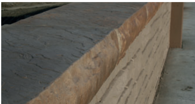
1a -- Simulated stone wall caps for a bridge project in Arvada, Colorado.
