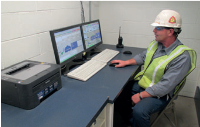
Figure 7 -- Vice President of Manufacturing Geoff Parrington checks the screens of the ACT PCS programmable control system used to operate the batching systems supporting both paving stone and retaining wall production operations.
